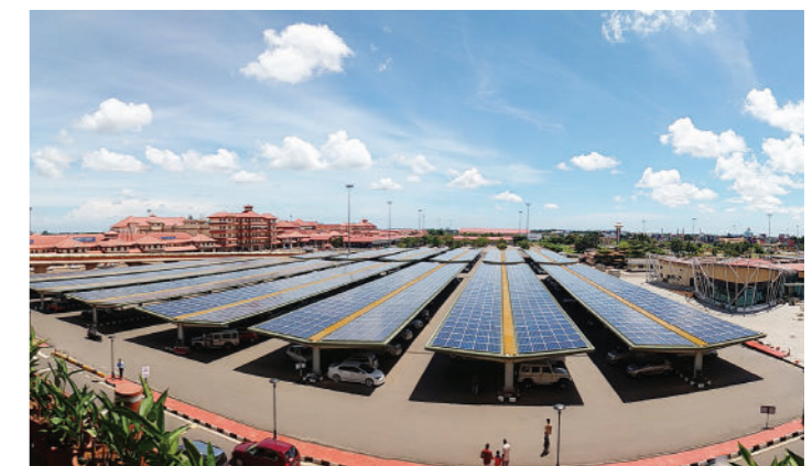
2.67 MW Carport installation at Cochin International Airport
