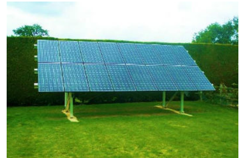
Ground-Mount Solar PV
